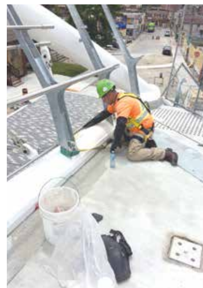
Paolo DiCarlo putting the finishing touches on the bottom cord of the John Street Pedestrian Bridge.
